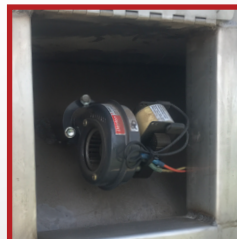
Two circulating fans
